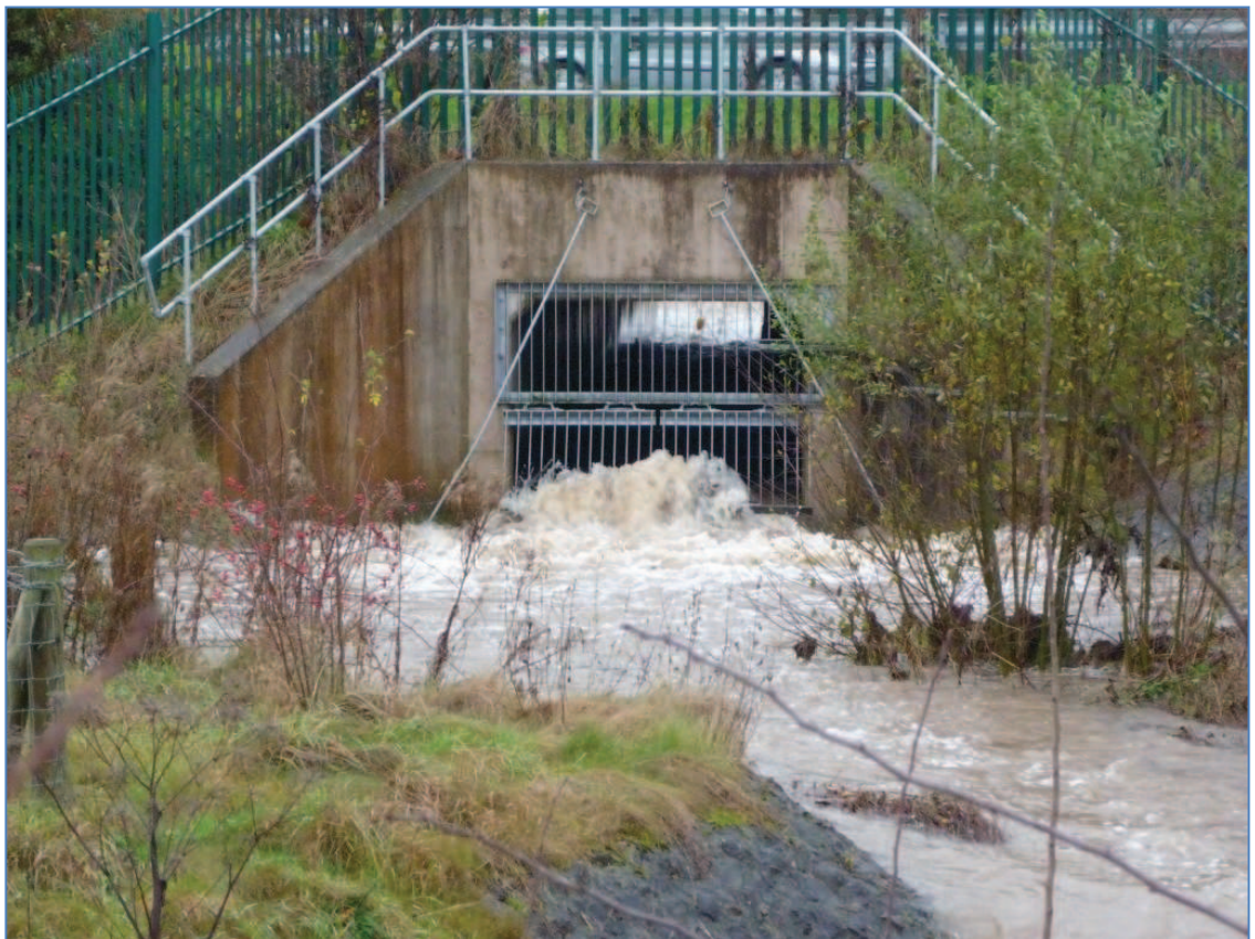
Plate 7 - Mwrog Flood Alleviation Scheme (November 2012)
