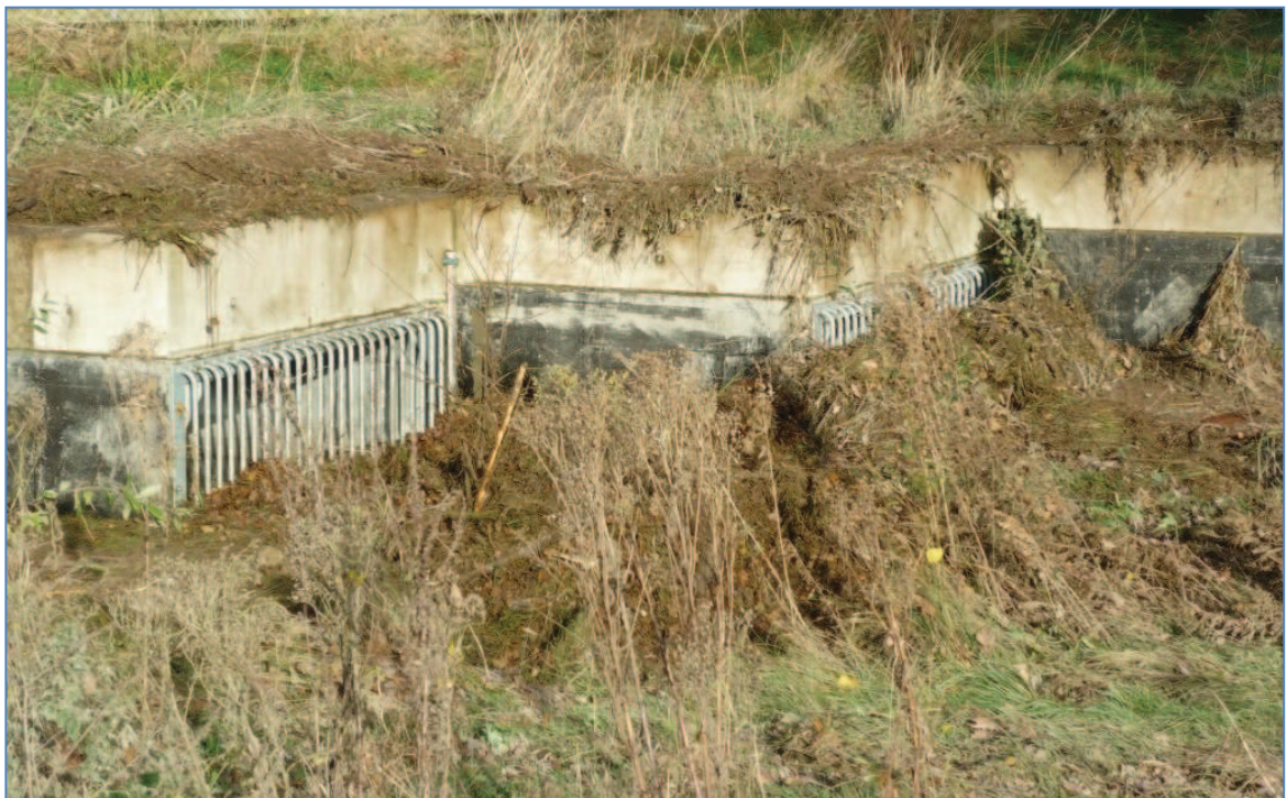
Plate 5 - Ruthin Link Road Culverts (Post November 2012 Flooding)
